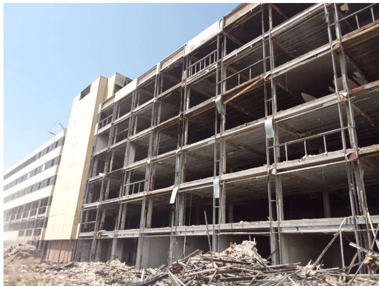
Plate 7: Maiduguri International Hotel perspective view showing damages cause by fire to non fire rated glass used in the hotel
