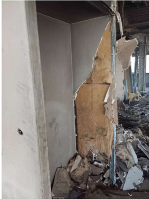
Plate 3: Hotel Internal partition wall constructed with Gypsum based with wool insulating material inside
