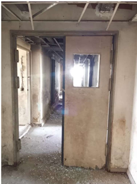
Plate5: Maiduguri International hotel double doors 1 hour fire rated door Source: author's field work (2024)
