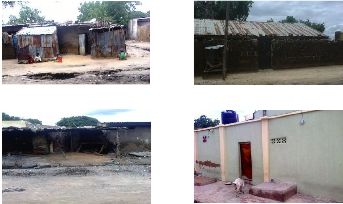
Figure 11: Structural Condition in Wulari Settlement
