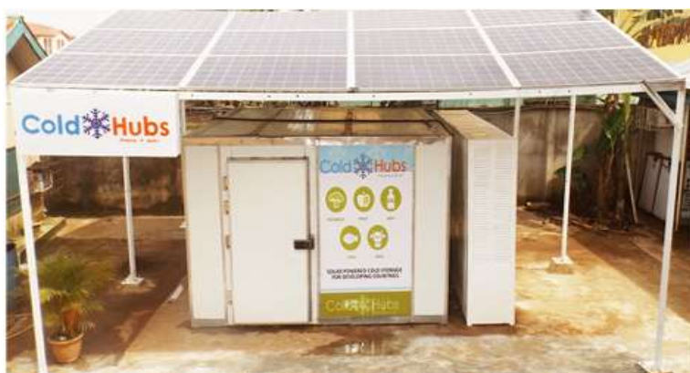
Figure 3: ColdHubs: a walk-in, modular, solar-powered unit for storing fresh produce in Nigeria
