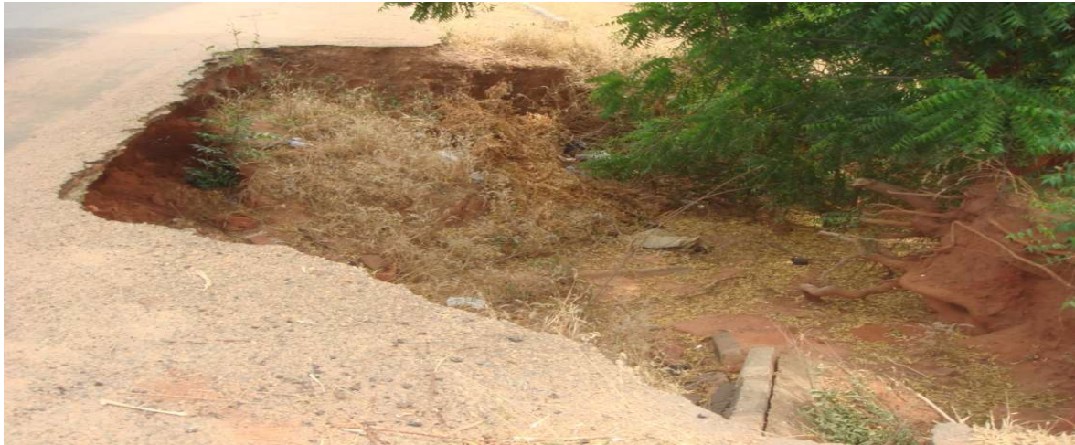
Plate 2: Gully undercutting regional road in Gona
