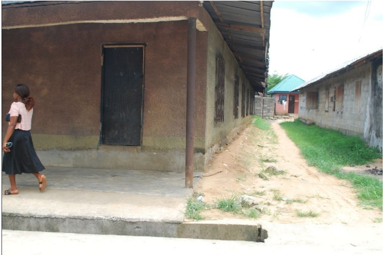
Fig. 3b: An Aged Painted Wall of Residential Building in the Study Area
