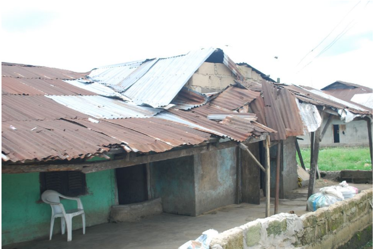
Fig. 4b: Blighted Residential Building on the Sampled Street
